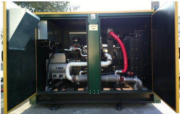
Fig. 3. Side-view photo of the cogeneration set CHP 64 kVA
