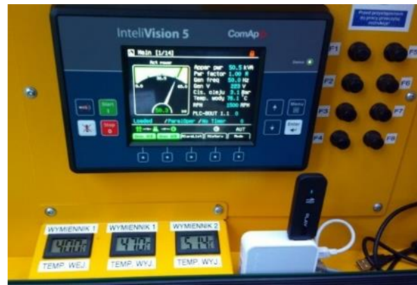
Fig. 5. Control panel during parameters reading. In the center, the main ComAp controller, below current water temperature readings at the heat exchangers. At the right – remote control module.
