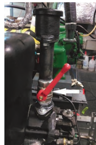
Fig. 1. A view of the inlet air duct supplying the engine: 1 – supply air control valve (degree of shutdown of the valve as during the laboratory
