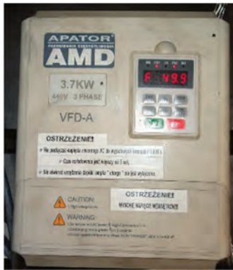
Fig. 7. The equipment used during testing: the electric inverter (coolant pump speed control)
