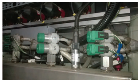
Fig. 3. Post-process gas fuel supply system of 12-cylinder engine
