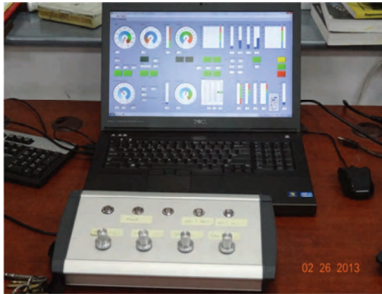
Fig. 4. General view of the control panel of the programmable controller
