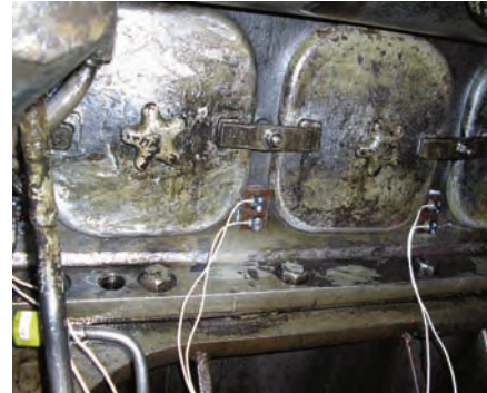
Fig. 2. Sensors mounted on an engine body
