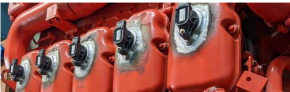
Fig. 14. Arrangement of ignition modules in the engine
