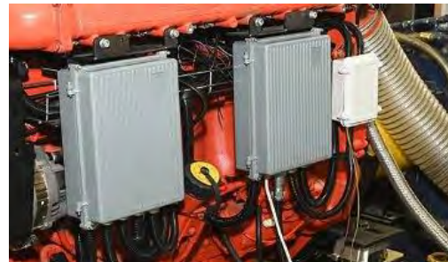
Fig. 16. Cassettes with the main engine control system
