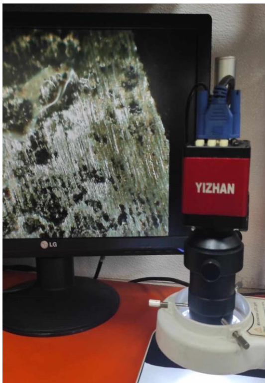
Fig. 6. Observation of corrosion on the hydraulic amplifier body
