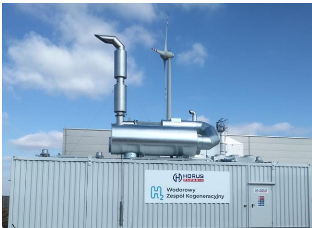
Fig. 4. The cogeneration unit with Perkins 4016-61TRS2 industrial gas engine equipped with the WUZG system at customer site in Gaj Oławski
