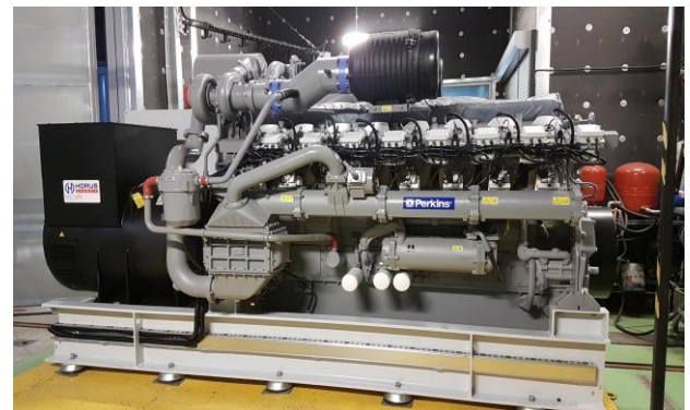
Fig. 5. The Perkins 4016-61TRS2 industrial gas engine is equipped with the specially developed system hydrogen-methane fuel system. The genset arrangement at Horus-Energia test facility
