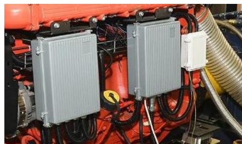
Fig. 16. Cassettes with the main engine control system
