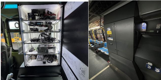
Fig. 19. Electrical cabinet on the wheel arch NA
